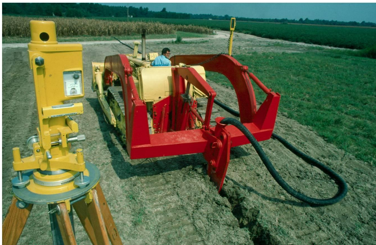
ARS Draintube Plow with Laserplane Automatic Depth & Grade-Control System Mounted on a D-7E CAT Installing 4-in. dia. Corrugated-Wall Plastic Draintube.
